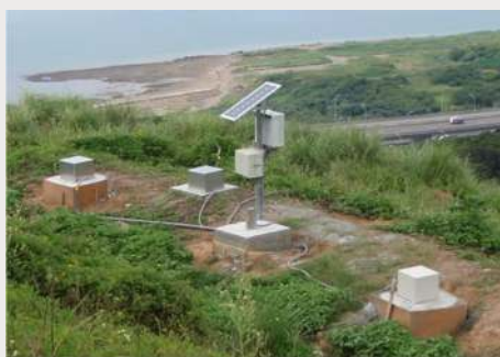
Instrumentation and monitoring for slope stability
