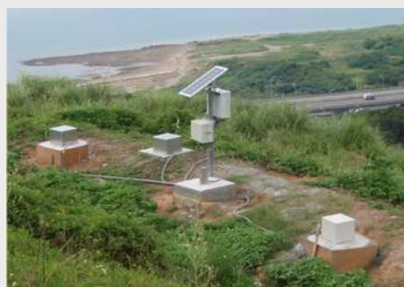
Instrumentation and monitoring for slope stability
