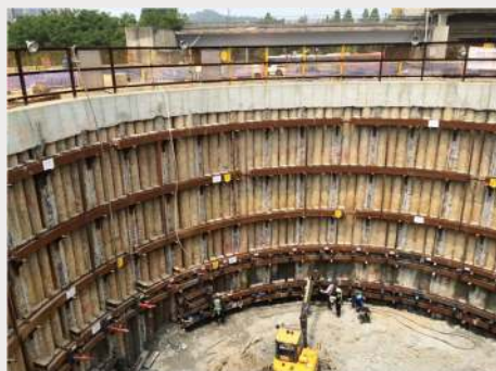
Instrumentation and monitoring for deep excavation
