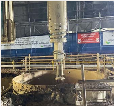
The SHAPE is lowered down into the bored hole with Kelly Bar
