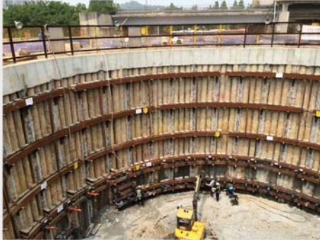
Instrumentation and monitoring for deep excavation
